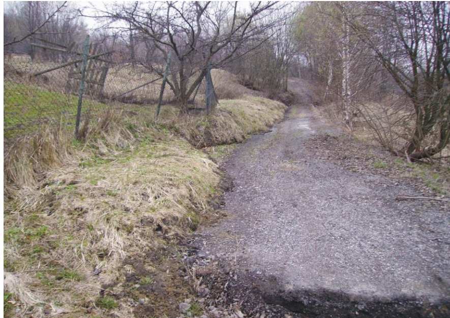
Figure 7. Narrowing of the local road due to sliding of the topsoil.
