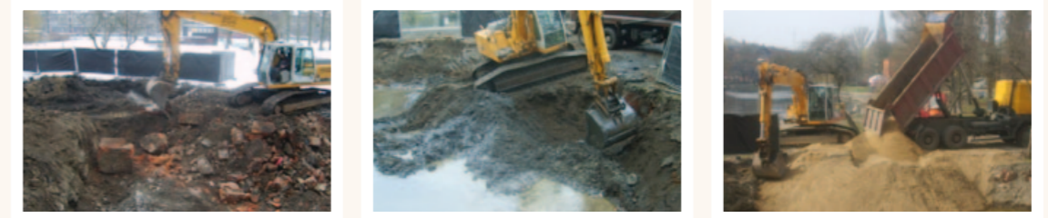
Fig. 12. Demolition of remains (A); excavation of contaminated ground (B); filling the trench with clean sand (C)
